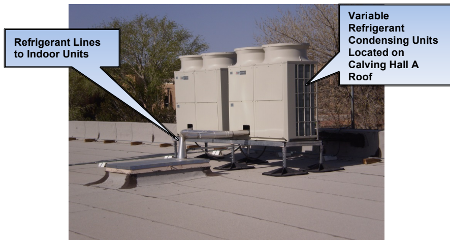
Figure 10: Calvin Hall VRF System Dedicated to Server Room
