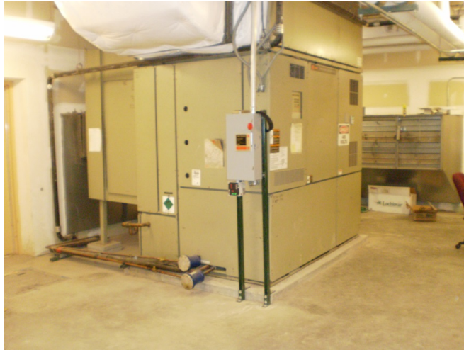
Figure 7: Zollinger Library Air Handling Unit
