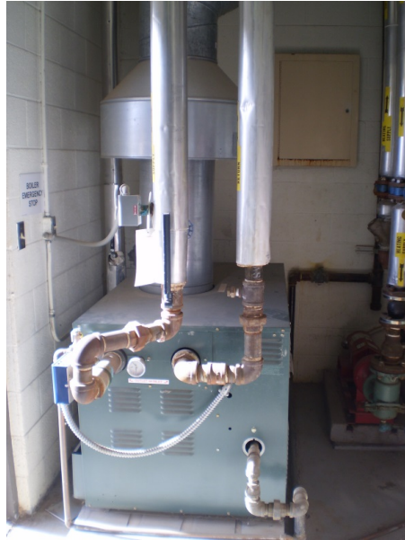
Figure 6: Gymnasium Heating Hot Water Boiler
