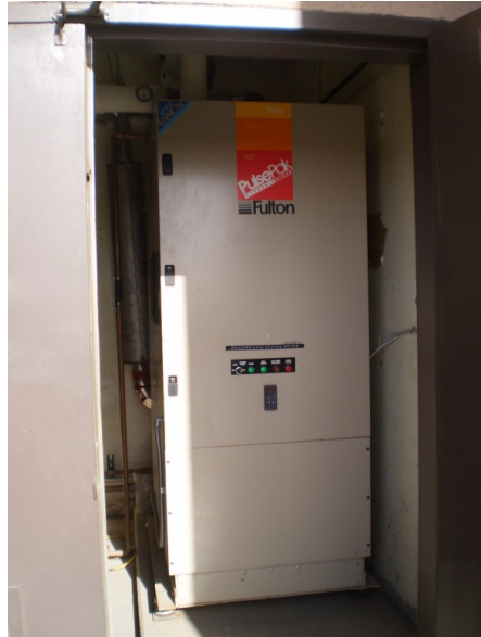
Figure 9: Calvin Hall A Boiler
