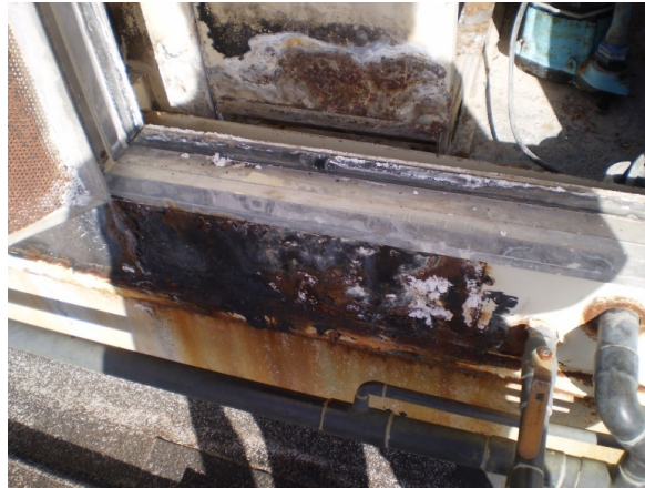
Figure 28: Calvin Hall C Rooftop Unit Rust and Calcium
