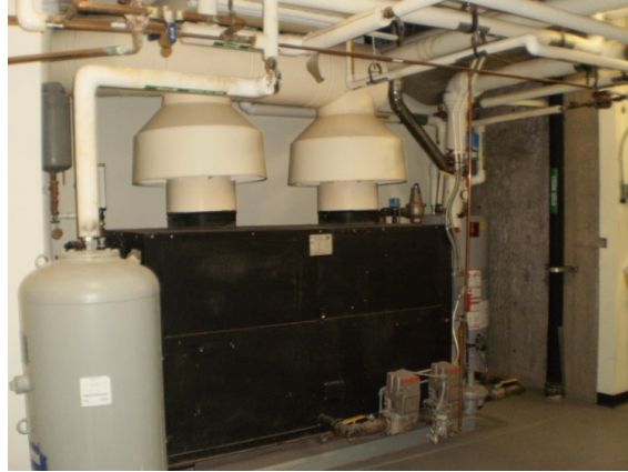
Figure 11: Calvin Hall Heating Hot Water Boiler
