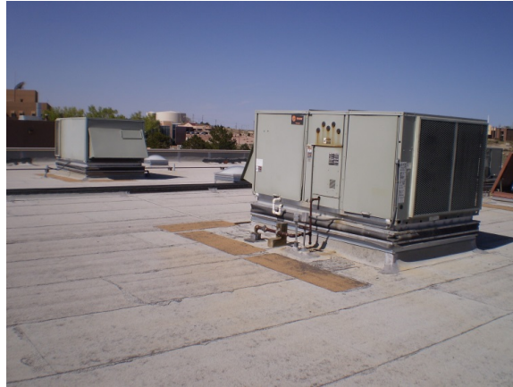
Figure 20: Health Careers Rooftop Units
