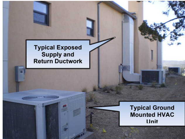
Figure 2: Lions Hall Package Ground Mounted HVAC Units
