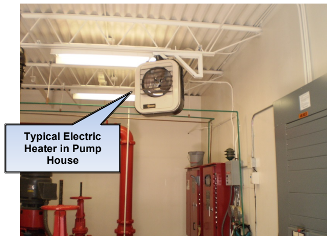
Figure 5: Pump House Electric Heater
