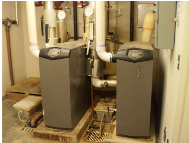
Figure 23: Student Services High Efficiency Boilers
