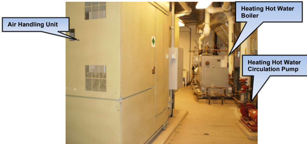
Figure 21: Health Careers 2 Mechanical Room
