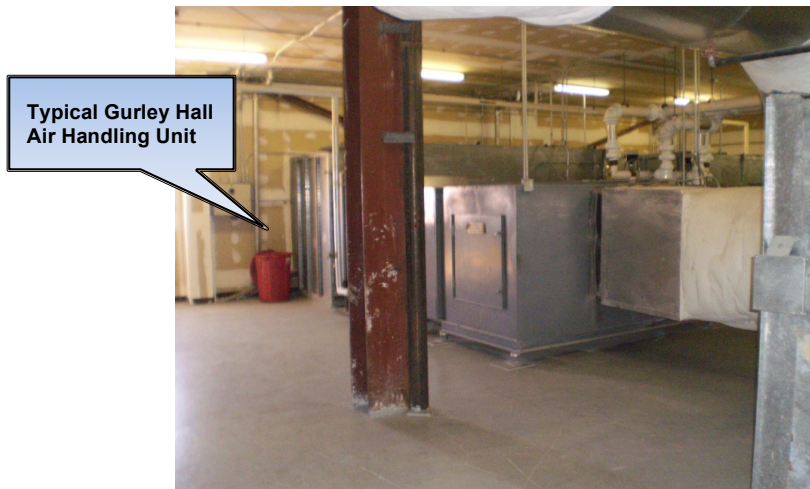
Figure 16: Air Handling Located within Mechanical Room
