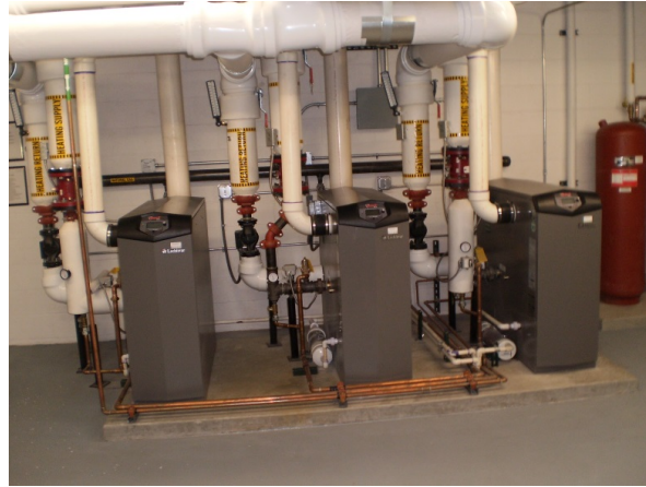
Figure 18: Career Education High Efficiency Boilers
