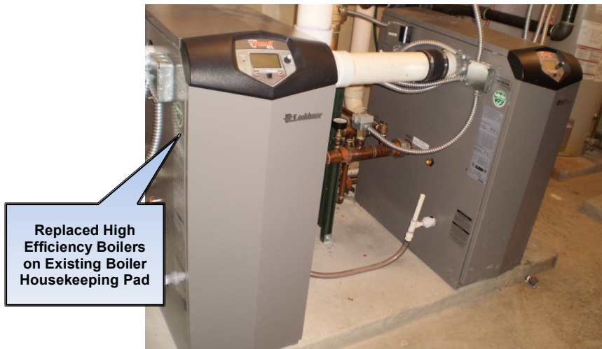
Figure 8: Zollinger Library New Heating Hot Water High Efficiency Boilers
